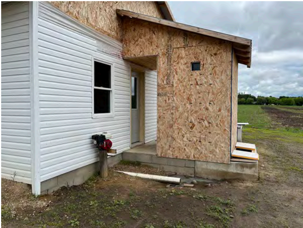
Noncompliant and unpermitted outhouse existing on the site
