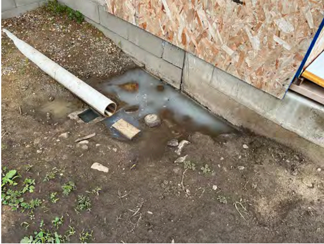
Discharged grey water existing on the site
